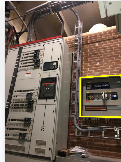
12 EMS Control cabinets
