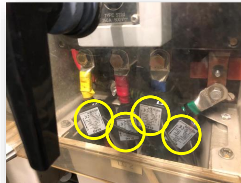
110 monitoring coils (>63 Amp)
